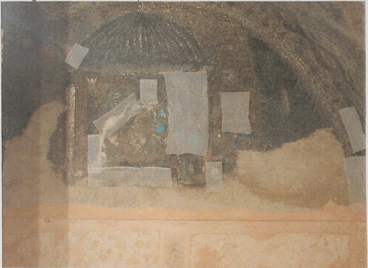
The decor is cracked. During a previous restoration, enamel tiles fragments were set into the plugging mortar.
