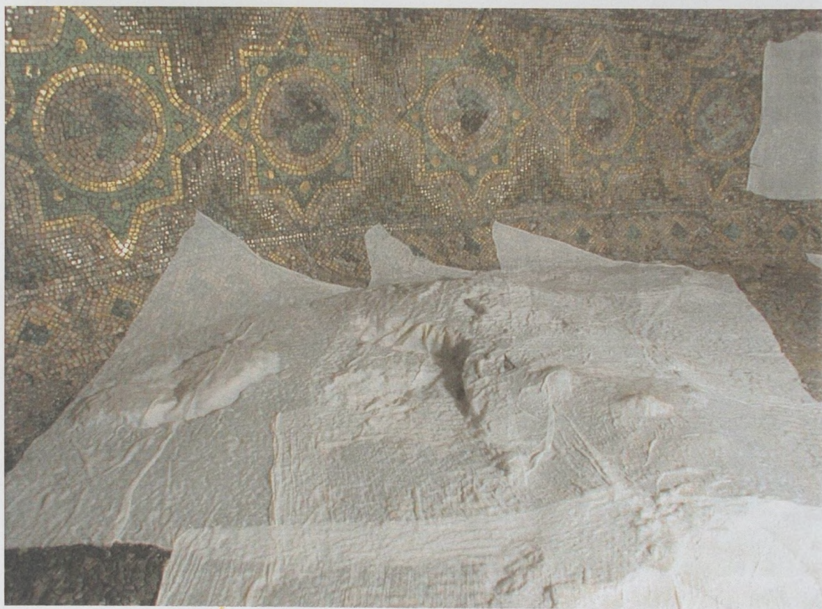
These cotton gauze sheets hold in the buckling areas, here in the north lunette.
