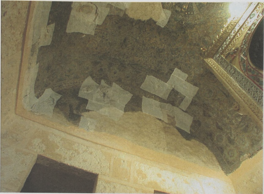
In 1997, the church was renovated; the lower part of the vault was edged, and cracks were filled with beige mortar. The grey cement fillings are older (before 1973).
